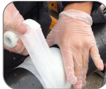
Wrap the bandage around the pipe several times with as much tension as possible. Ensure you go 50mm to either side of the leak
