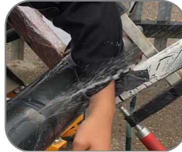
Wrap the amalgamating tape to the side of the leak. Ensure the tape is wrapped as tightly as possible
