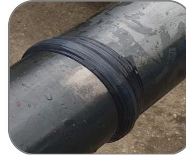
Wrap the amalgamating tape over the leak, applying as much pressure and tension on the tape
